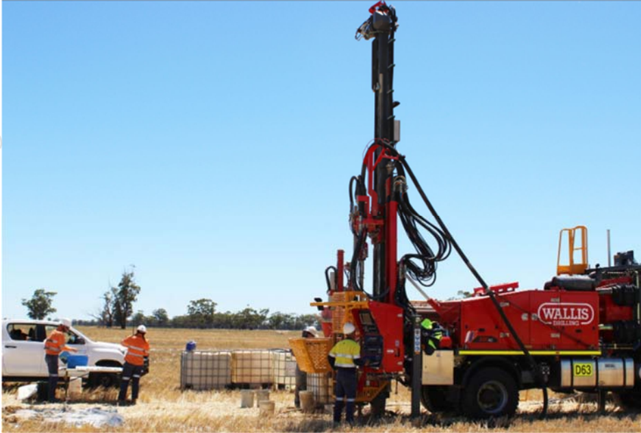
Figure 4 Air Core drilling at Caledonia. A larger rig – capable of drilling significantly deeper holes - has been mobilised to drill the northern, deeper targets.
