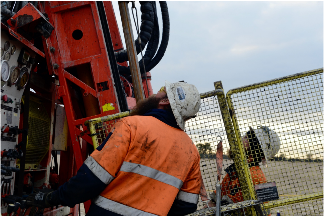
Fig1. Completing the last diamond drill hole for the current Wildwood programme, April 2021.
