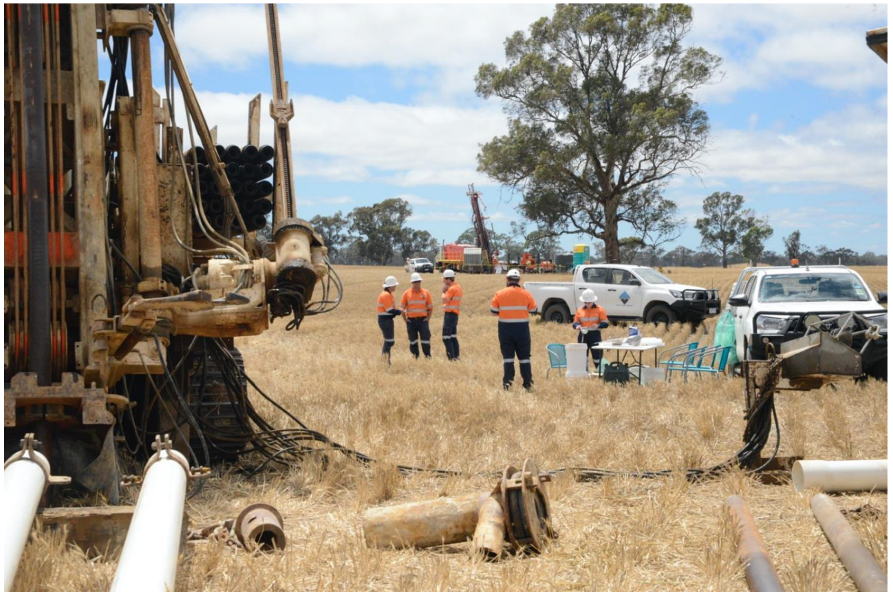
Fig5. RC rig in the foreground, NSM field team preparing to sample RC samples and diamond drilling rig in the background. January 2021
